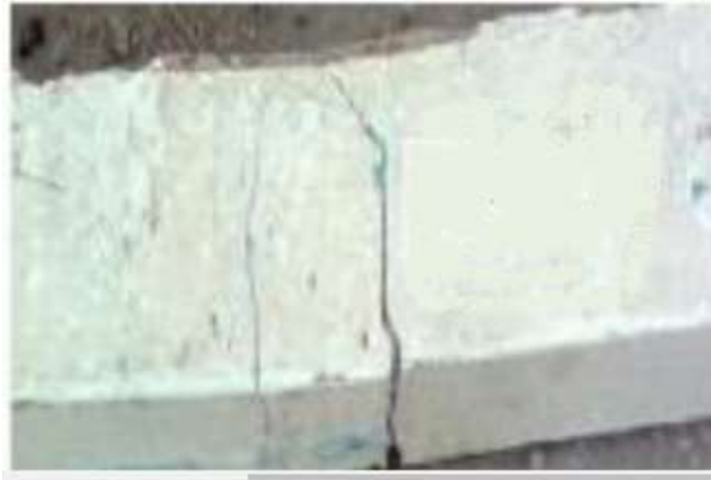
Fig 5. Pattern of crack in Steel Reinforced concrete slab
