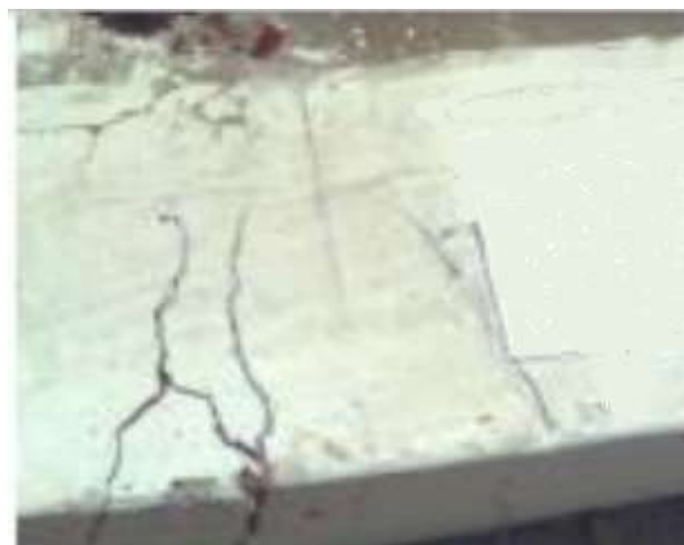
Fig 6. Pattern of crack in Bamboo Reinforced concrete slab
