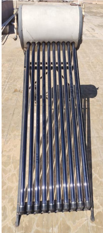
Figure 3. Evacuated tube solar water heating system
