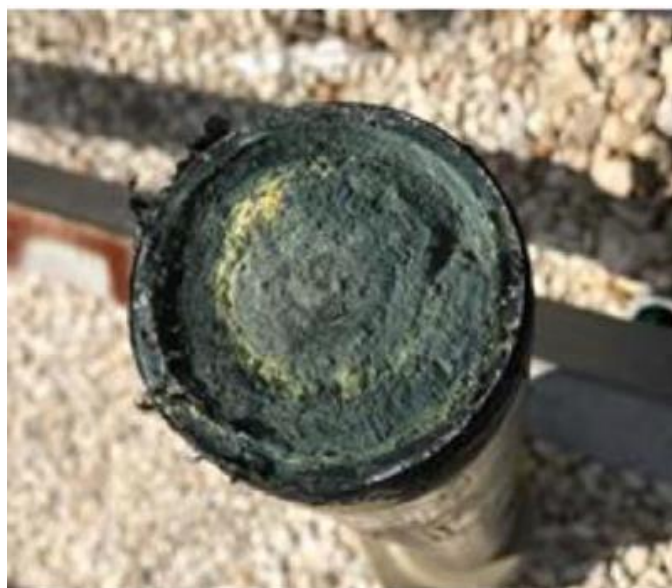
Figure 2. Drain pipeline plugged with amorphous dithiazine.
