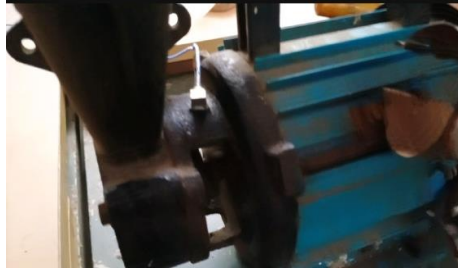
Figure 1. Induction motor chosen for vibration monitoring
